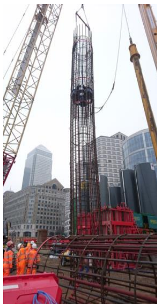
Figure 6. Lifting the O-cell cage to vertical ready for installation in the pile bore (Canary Wharf).
